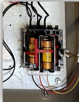
Fused Disconnect Switch
